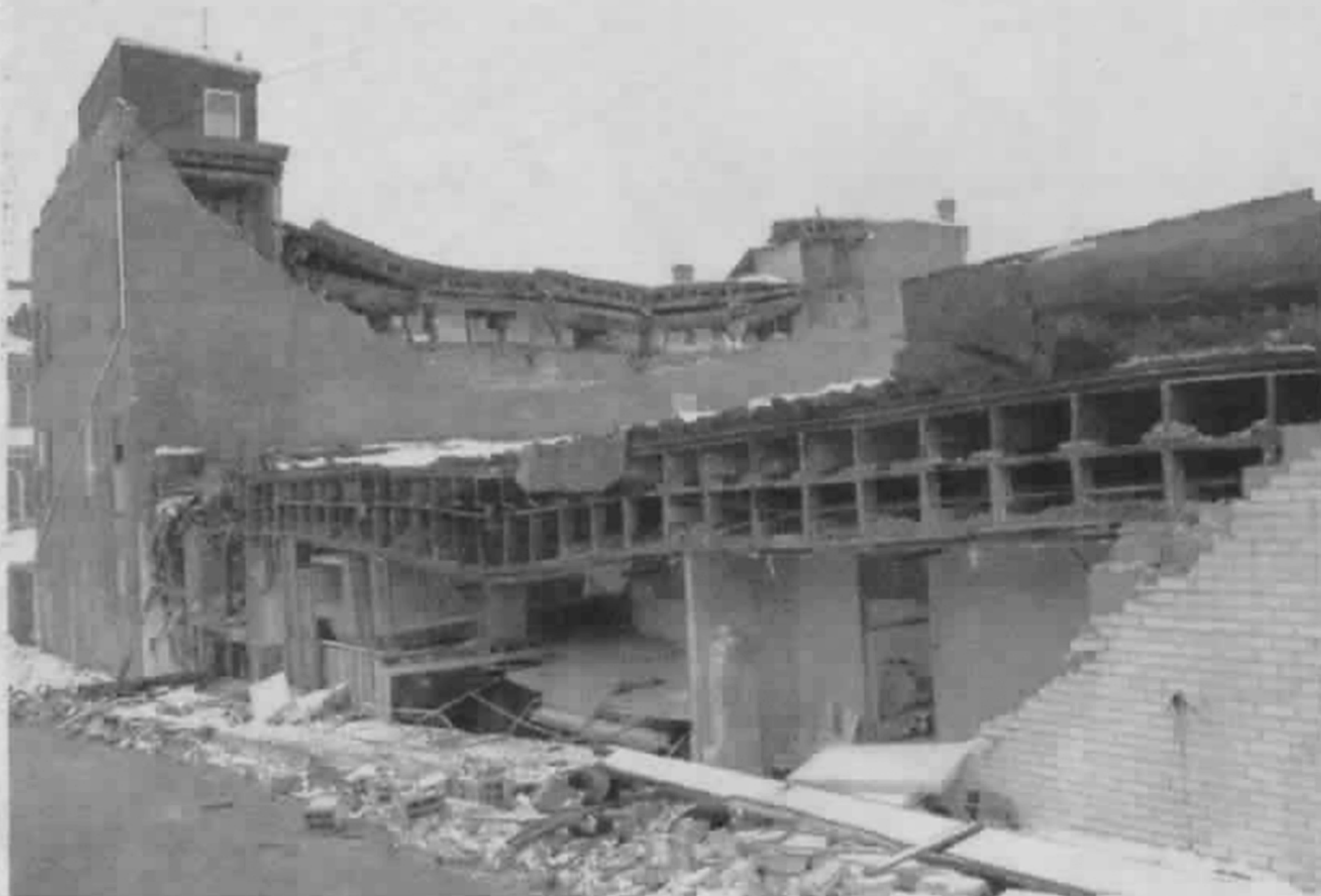
The aftermath of the roof collapse which killed three in Pittsburgh
